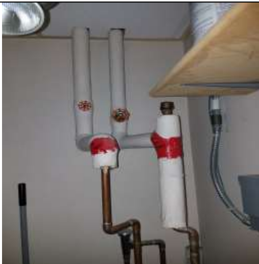
Janitor closet 2071, asbestos pipe fittings
