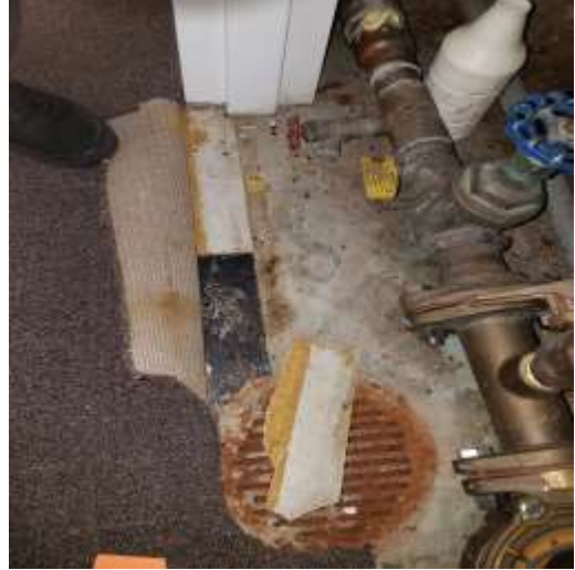
Kindred floor tile/mastic under carpet, asbestos
