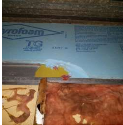
Vacant space glue streaks, not asbestos
