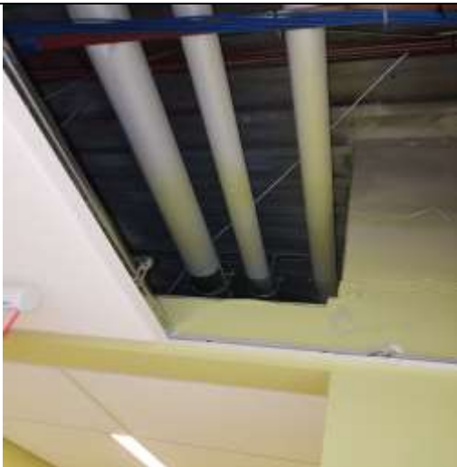
New fiberglass insulated pipes in plenum
