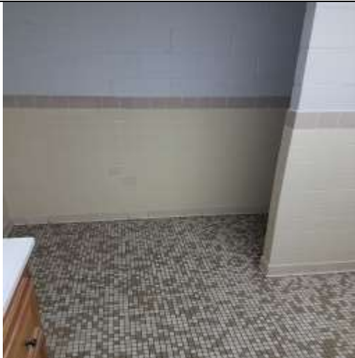
Lead paint glaze in bathroom ceramic wall
