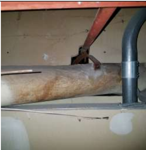
Asbestos mud on drain hanger
