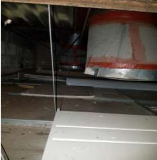
Red seam on exhaust, not asbestos
