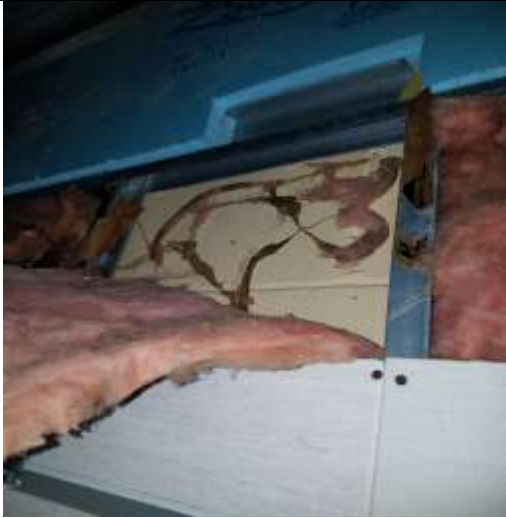
Vacant space glue streaks, not asbestos
