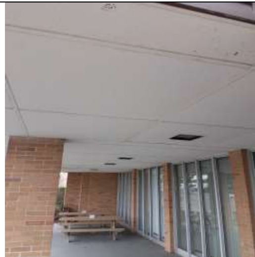
Asbestos ceiling panels at rear entrance
