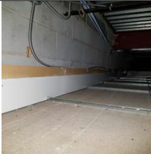
S/E vacant section outer wall, asbestos JC
