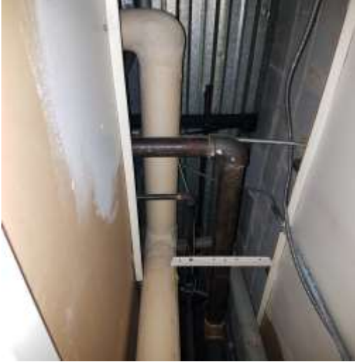
Kindred space, asbestos fitting
