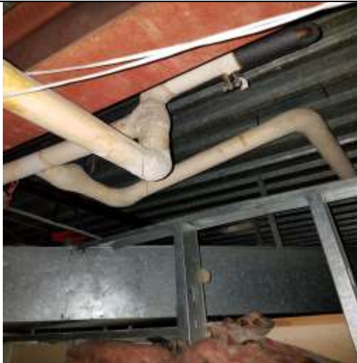
Asbestos pipe fittings in cafeteria plenum
