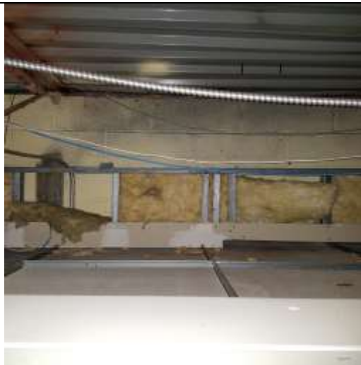
Newer gypsum and JC in vacant section
