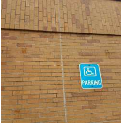
Wall expansion, not asbestos
