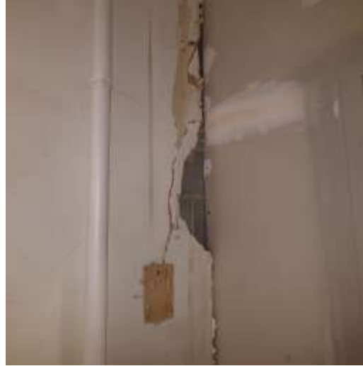
South wall with damage, asbestos
